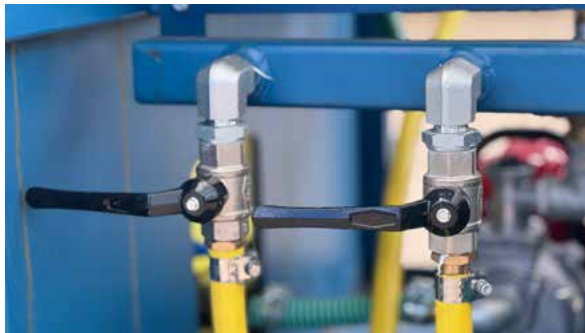
SPRINKLER & HOSE VALVES
